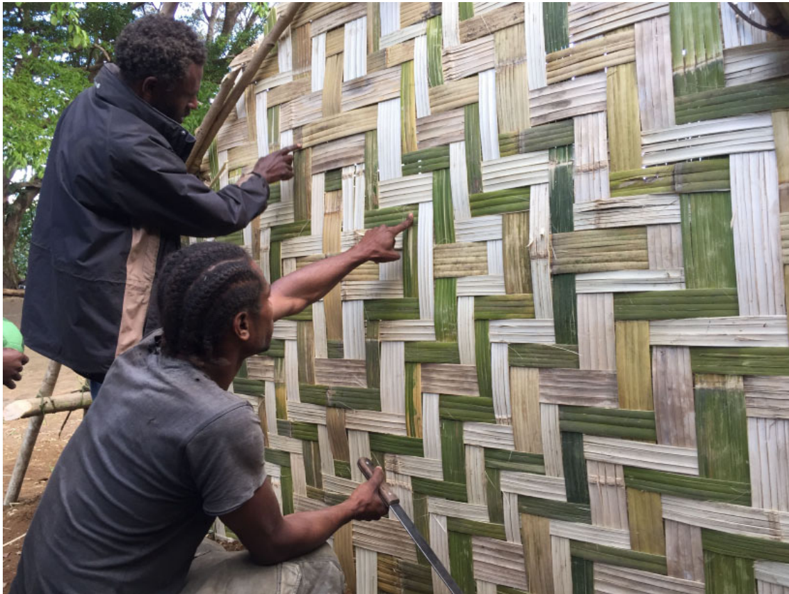
Figure 5. Building a Nafe cyclone house made entirely of plants, used to protect islanders from dangerous storms and also built by the tupanas for the sun as a holy house used for magic.
